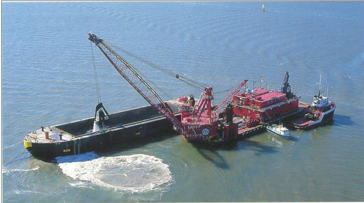
Figure 12-16: The largest clamshell grab used in dredging, the Chicago, in full operation.
